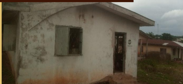
Situation Before Osun CSDA Intervention
