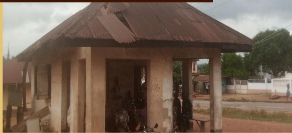
Situation Before Osun CSDA Intervention
