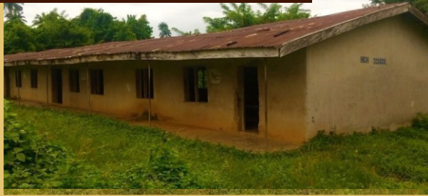
Situation Before Osun CSDA Intervention
